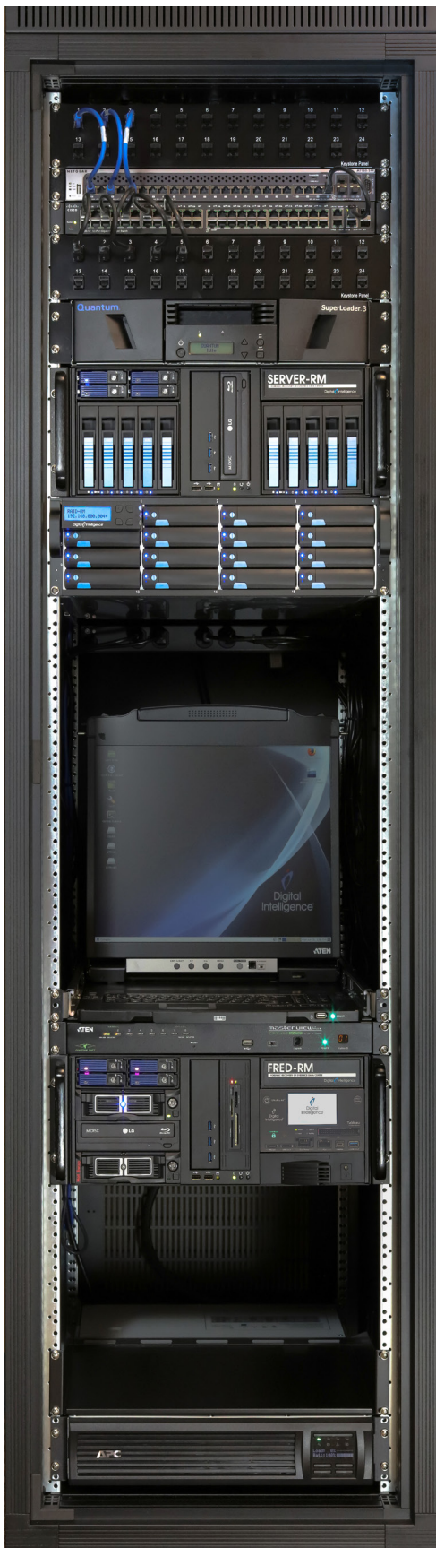
FREDC showing (from top): network switches, tape subsystem, Server-RM, RAID-RM, monitor and keyboard, KVM switch, FRED-RM and UPS
